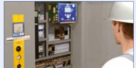
Control system assembly
